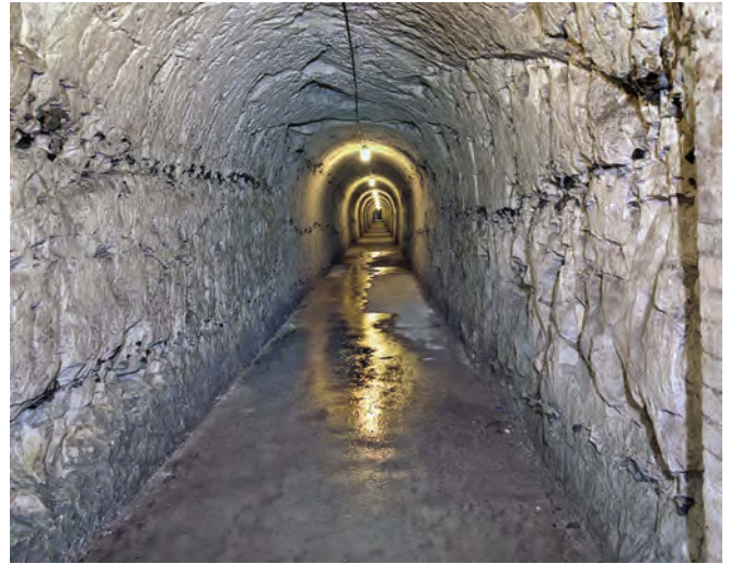
Looking northwest along the tunnel to the western caponier from the bottom of the spiral staircase. Photo Nick Catford
